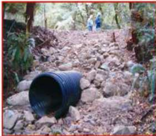
Drainage Control System (Konkan, Maharashtra)
