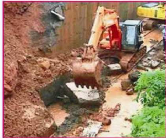
Photograph (D) Retaining wall collapse on railway track in konkan region
